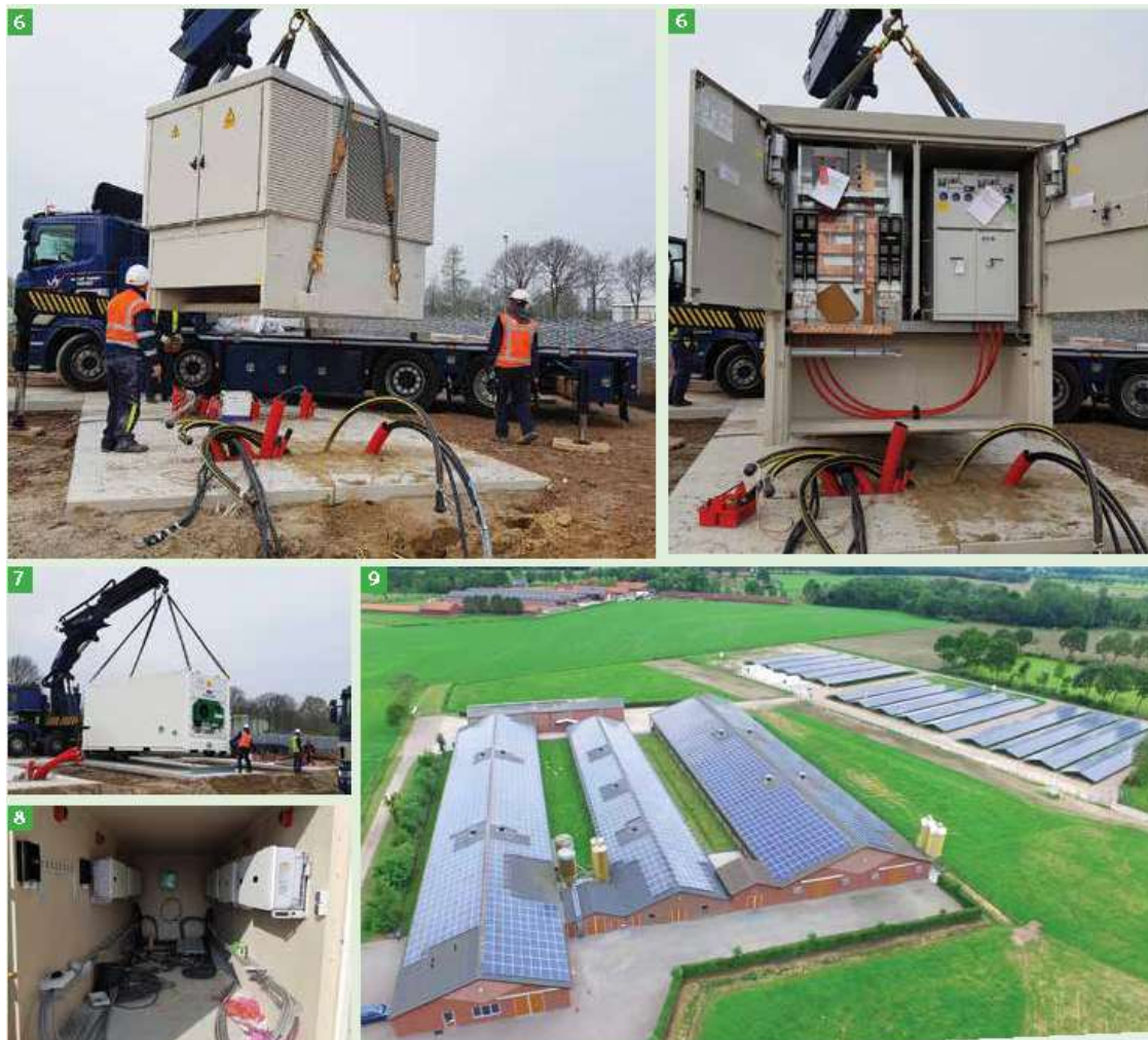
Figure 10: The 612 KWh battery of Weert Energy and solar park 16
